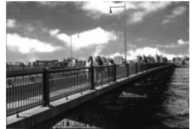
The Harvard (Mass. Ave.) bridge provides an important link between Cambridge and Boston. Without well-located bridges over rivers, railroad tracks, and highways, many trips would be too long to walk. MassHighway reconstructed the Mass. Ave. bridge in the late 1980s with increased sidewalk width.
