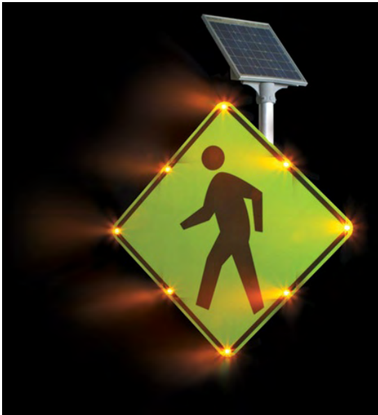
Figure 8: Another pedestrian button actuated flashing sign (W11 MUTCD) Rectangular Rapid Flashing Beacons – RRFB
