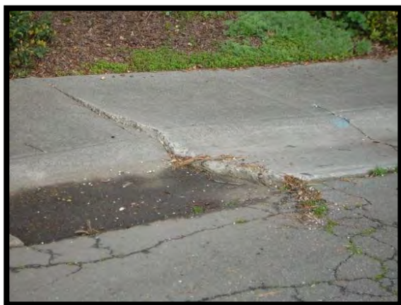
Figure 6: Example of short curb reveal
