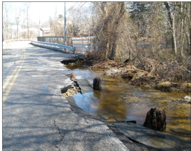
Figure 3.22: The Bridge Street Bridge spanning the Matfield River in Bridgewater was damaged and closed due to extreme flooding in March, 2010.
