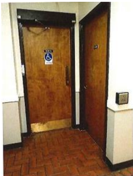
Figure 39: Non-compliant restroom signage in Town Hall
