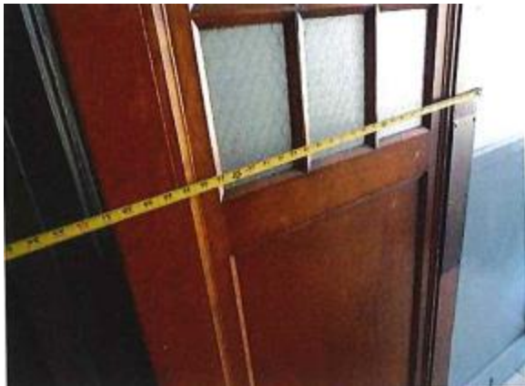
Figure 51: ADA non-compliant door width
