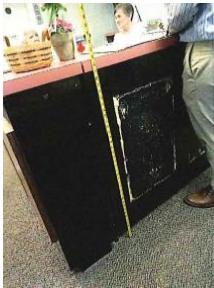
Figure 56: The COA Non-ADA compliant service counter
