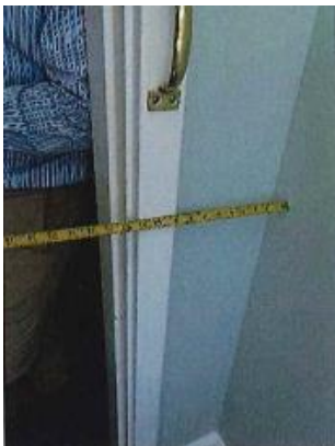
Figure 55: The COA interior doors
