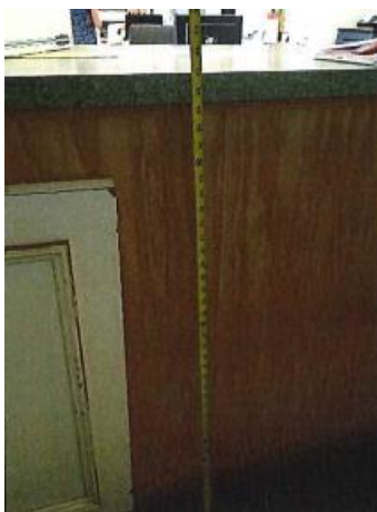
Figure 41: Non-compliant counter height
