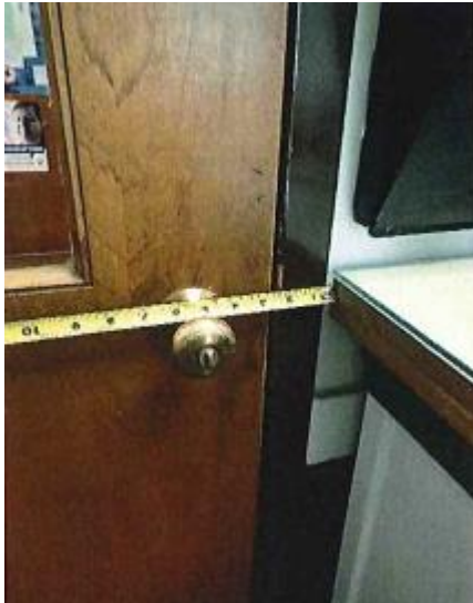
Figure 40: Non-compliant door hardware at Town Hall
