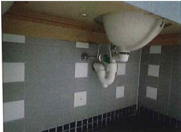
Figure 60: Missing insulation at hot-water piping below lavatory, Men's room
