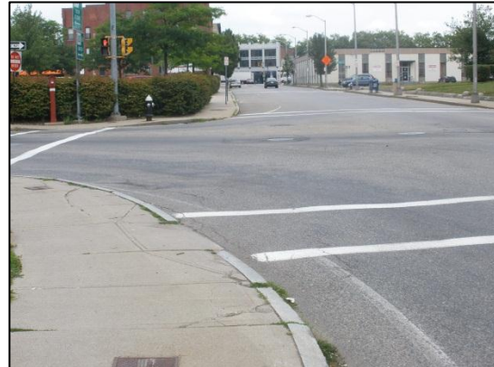
Broken sidewalk at the Warren Avenue/Belmont Street intersection from truck wheels jumping the curb onto the sidewalk (from right turns).
