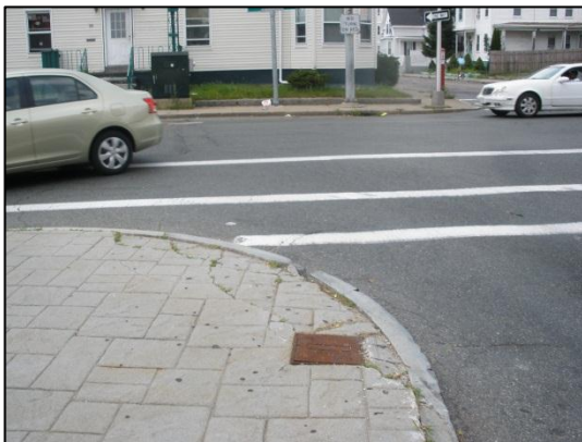
Broken sidewalk at the Legion Parkway/Warren Avenue intersection from truck wheels jumping the curb onto the center median (from left turns).
