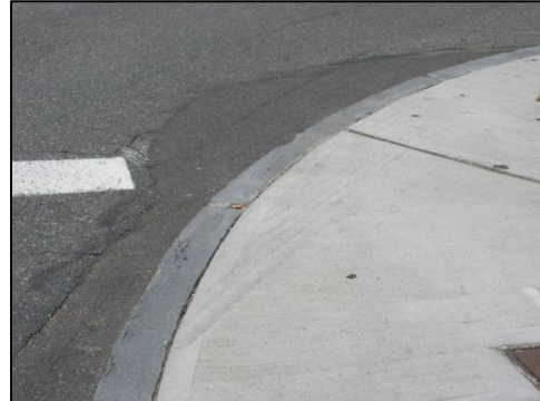
Truck tire marks on sidewalk at the Main Street/Crescent Street intersection from truck wheels jumping the curb onto the center median (from right turns).
