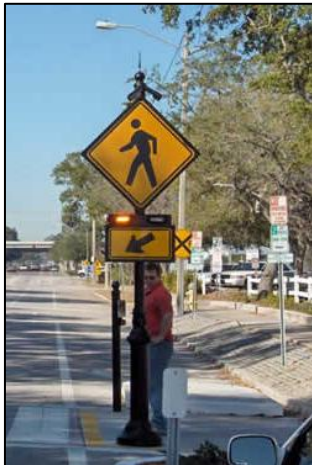
Rapid Rectangular Flashing Beacon
