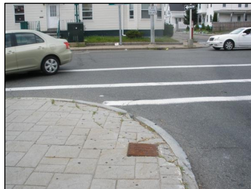
Median and curb at Warren Avenue and Legion Parkway broken due to truck turns
