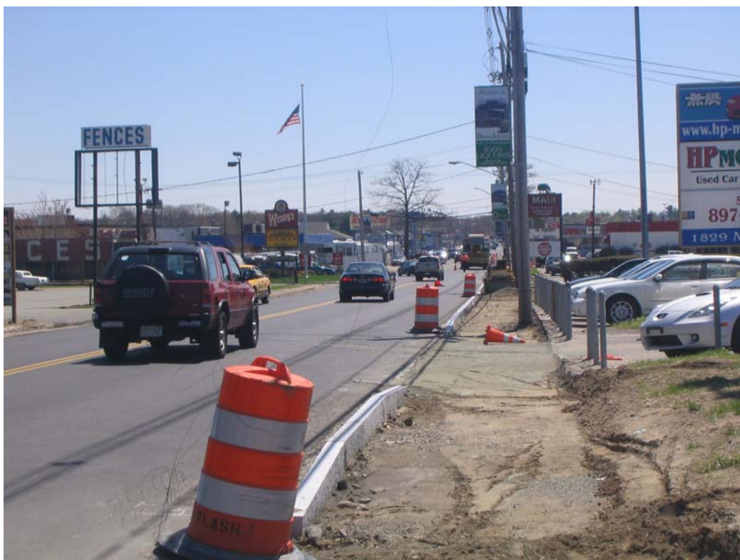
Pavement rehabilitation on Route 28 south Brockton (to extend through West Bridgewater to the Bridgewater line.)
