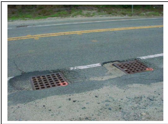
Figure 7: Pavement deterioration around catch basin
