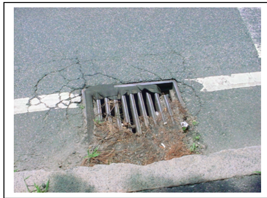
Figure 8: Dirt and other debris clog a deteriorated catch basin cover
