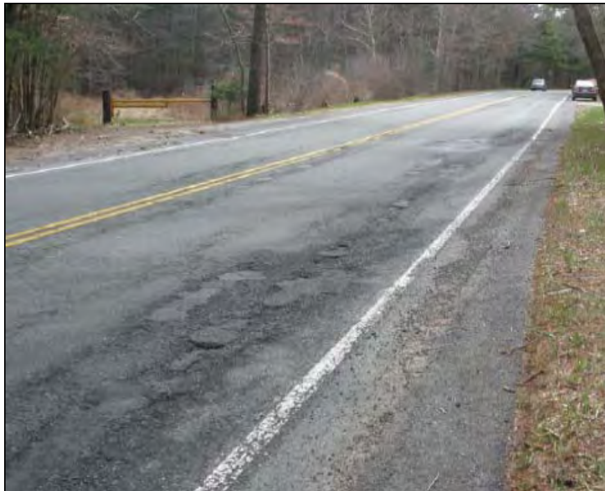
Route 58 Pavement Conditions in Halifax near Palmer Mill Road (Poor conditions).
