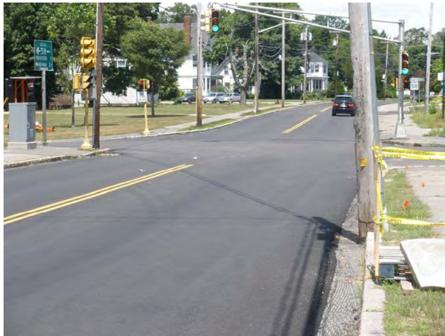
The Route 58/Route 139 intersection showing resurfacing of Route 58 under the Abington PWED improvement project.
