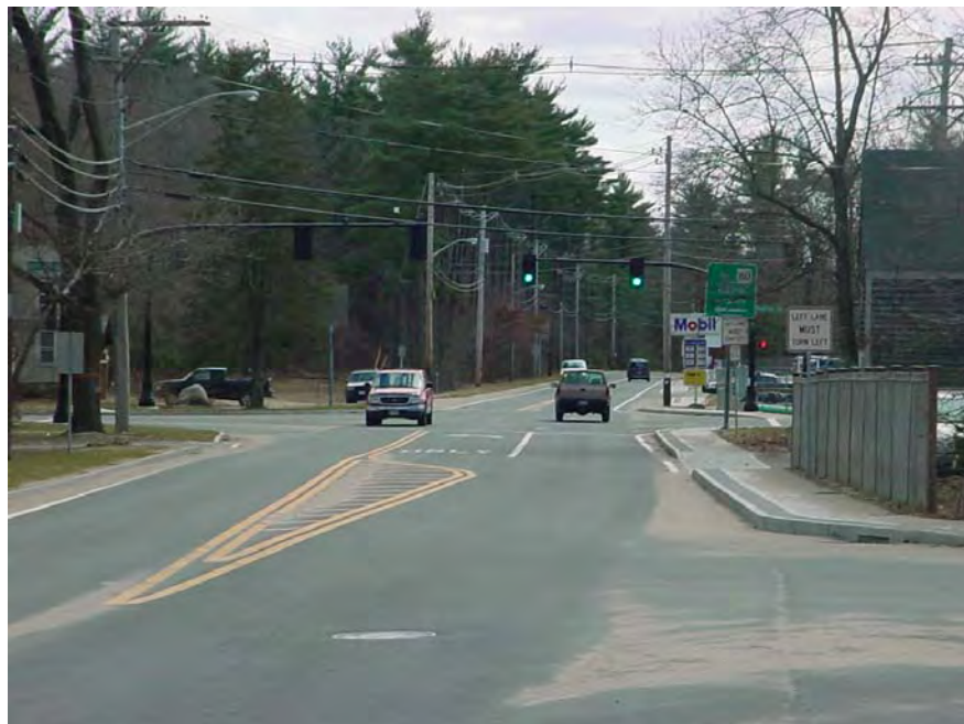
Route 58, Plympton at showing completed improvements for Route 58 that include re-stripping, pavement resurfacing, and installation of a traffic signal at the Route 58 Parsonage Road/Mayflower Road intersection.
