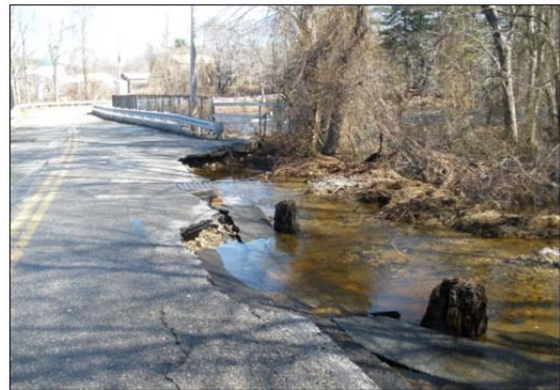
Figure 8-13: The Bridge Street Bridge spanning the Matfield River in Bridgewater was damaged and closed due to extreme flooding
