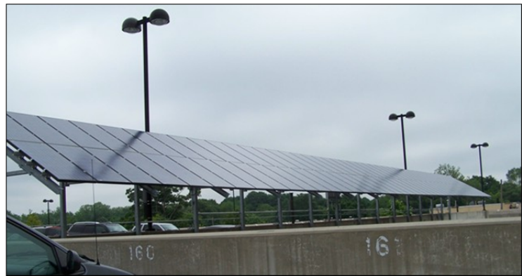
Figure 8-19: Solar Panels on the BAT Intermodal Centre in Brockton
