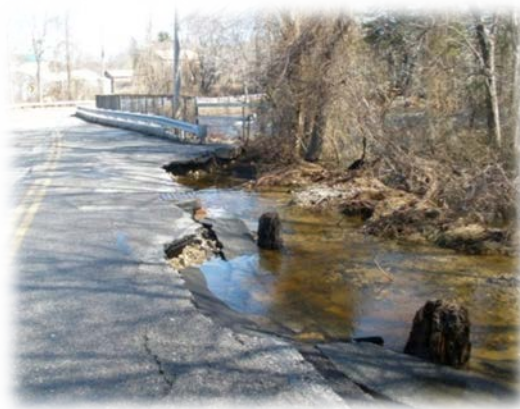
Figure 8-3: The Bridge Street Bridge at the Matfield River in Bridgewater as a result of extreme flooding in March, 2010.
