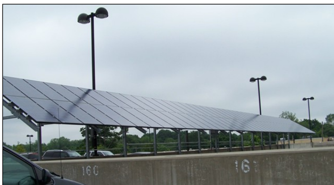
Figure 8-4: Solar Panels on the BAT Intermodal Centre in Brockton
