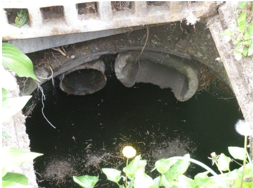
Figure 3. An example of a typical catch basin, showing concrete and metal pipes.
