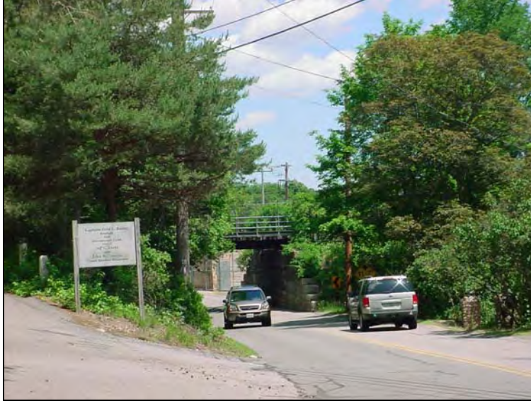
The MBTA Bridge over Landing Road at Captain Bailey Park looking northbound
