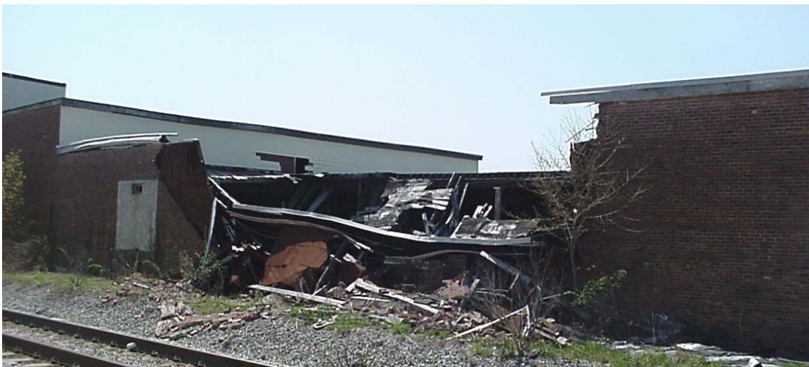
South Hanson - Deteriorated former Ocean Spray warehouses south of the tracks, proposed for redevelopment
