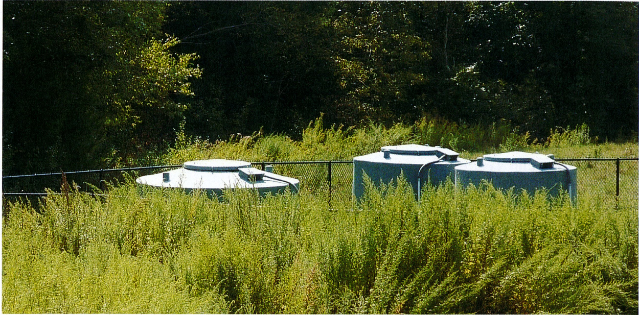
Bioclere wastewater treatment system to the rear of Roche Bros. Plaza
