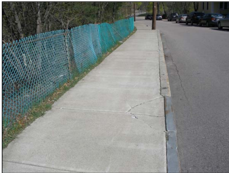
Fence along MBTA right of way and Sullivan Street in disrepair
