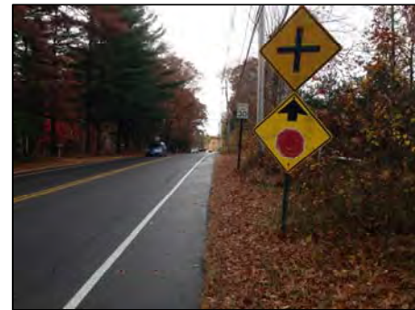
“Stop Ahead” signage on Chestnut Street westbound is faded, and intersection warning signage is inappropriate.
