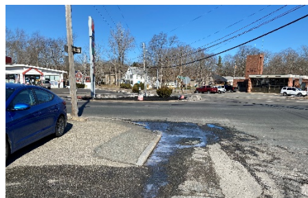
Image 2: Image shows poor pedestrian connectivity through intersection, and ponding of water on southwest corner.
