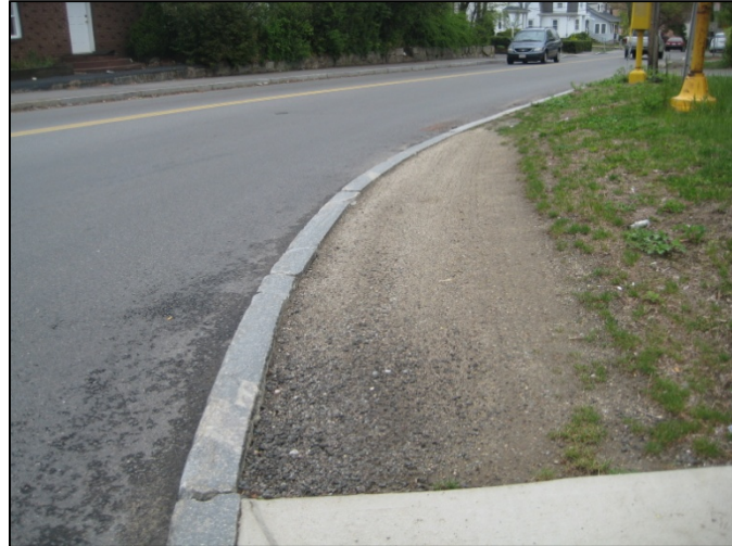
Tire tracks over curb/sidewalk at southeast corner from large trucks.
