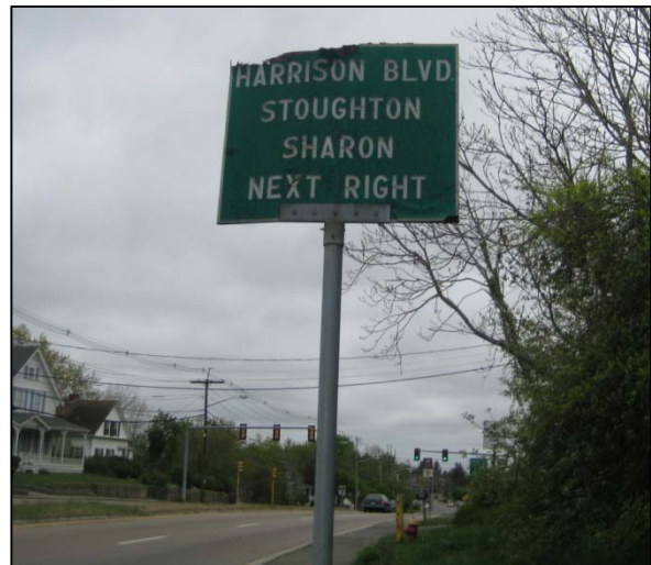
Guide sign along Route 28 southbound is in poor condition.
