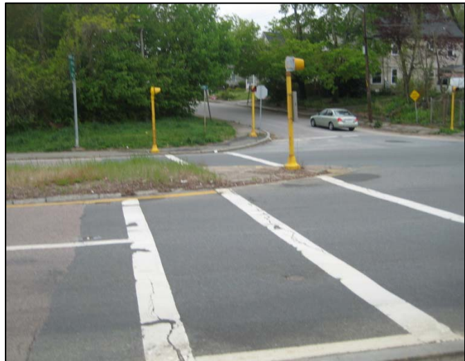
Stop line pavement markings at Route 28 Northbound and Southbound approaches add to driver confusion.
