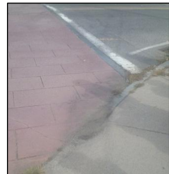
Signs of ponding on the crosswalk
