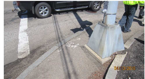
Image 2: Sidewalk obstructed by signal equipment
