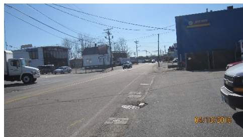
Image 3: Poor access management along Belmont Street
