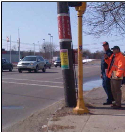
Utility pole located near the curb line and leaning towards the travel lane.
