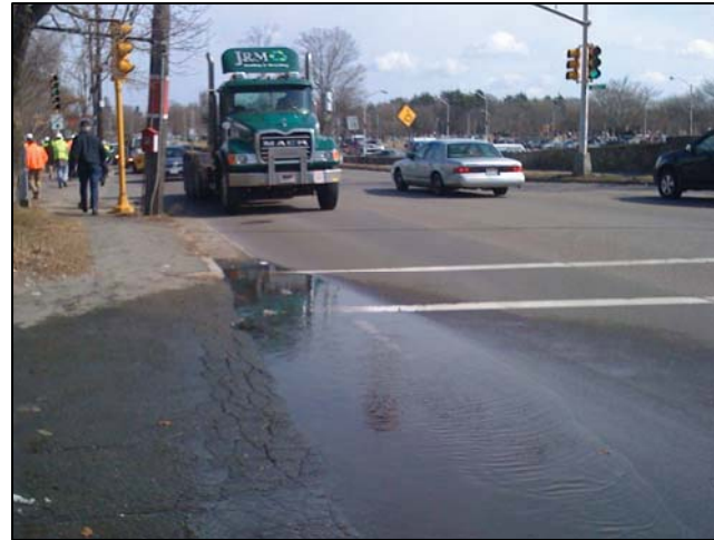
Drainage issues along Belmont Street
