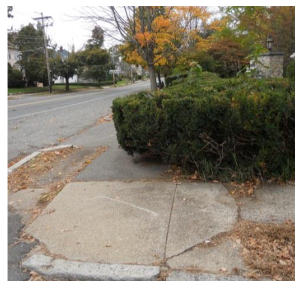
Vegetation encroaching on existing sidewalk
