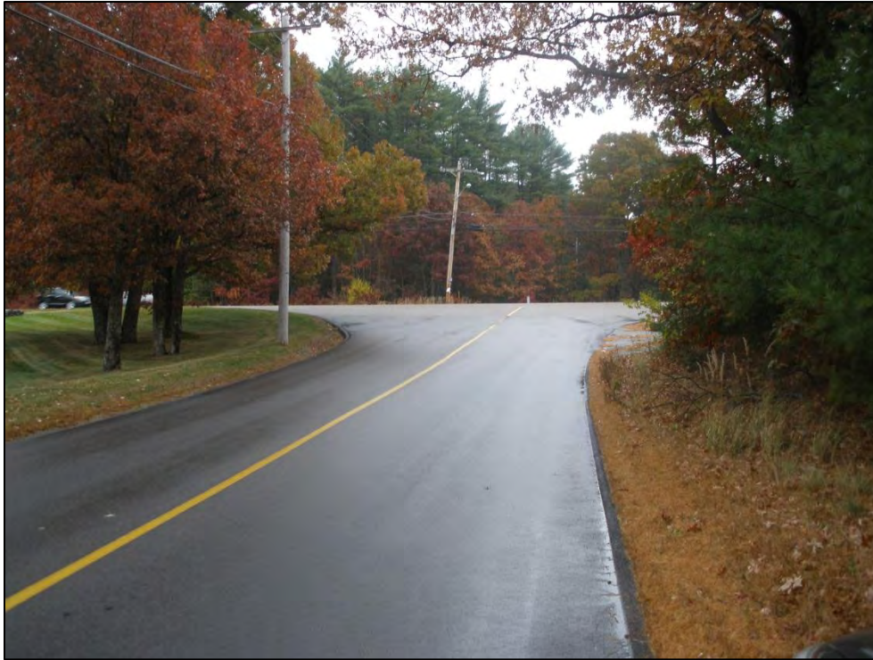
Franklin Street minor street approach to the Franklin Street/Main Street (Route 27) intersection shows a lack of stop sign and stop line and wide mouth as it intersects Main Street (Route 27)
