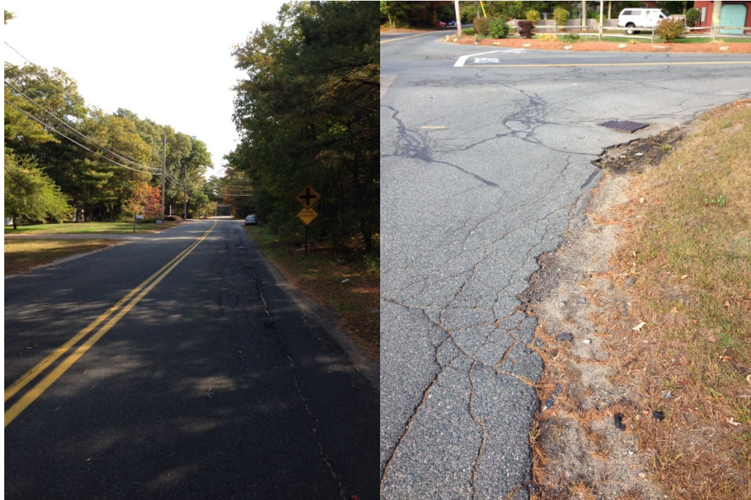
Figure 6: Photos show pavement distress on approaches to intersection
