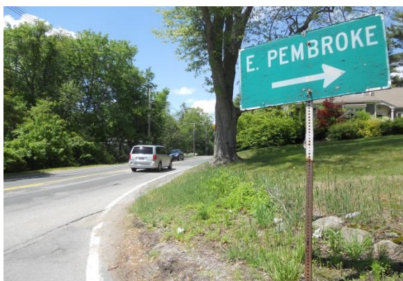
Tree on northeast corner restricts visibility (looking north)
