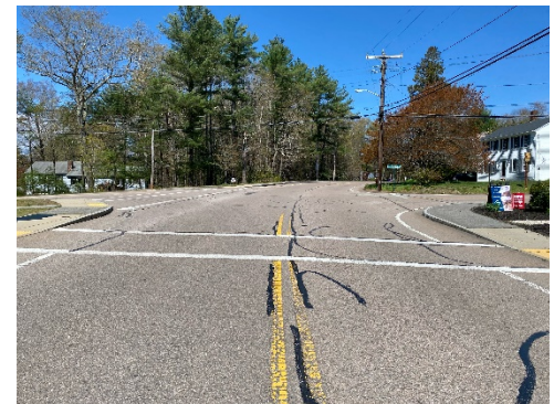
Image 1: Curvature of Route 27 restricts sight lines to the west. Utility pole on northwest corner is vulnerable to traffic.
