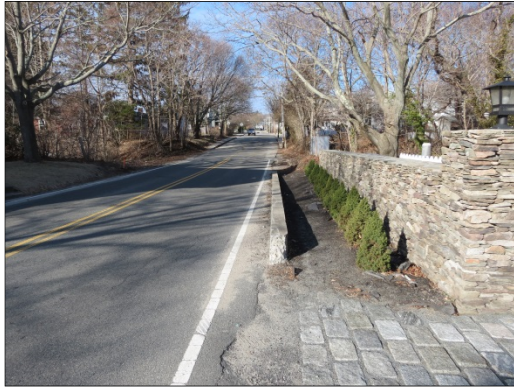
Curb showing damage in front of #32 Nelson Street
