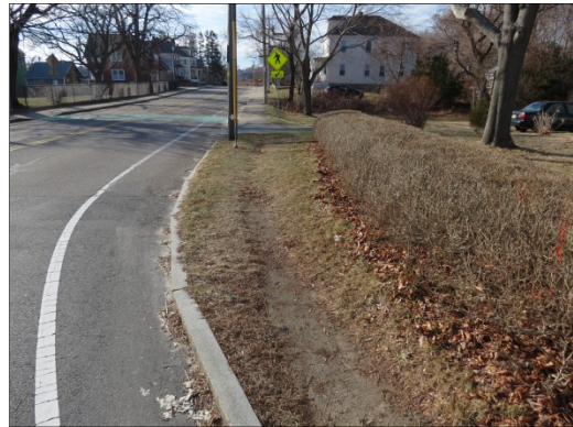
Inside of curve showing no sidewalk but clear indication of pedestrian use
