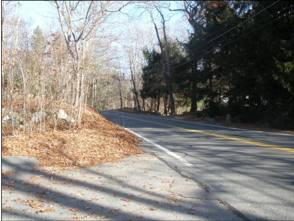
Bay Road southbound approach to Boulder Lane (looking northbound from Boulder Lane toward slope and curvature away from the intersection). This photo shows the limited visibility for vehicles exiting Boulder Lane, preventing motorists exiting Boulder Lane from safely exiting the road and entering Bay Road.
