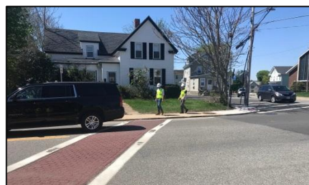
Curbing on the southeast corner of the intersection lacks ADA ramps for the crosswalk at the Canton Street (Route 27)/School Street intersection.
