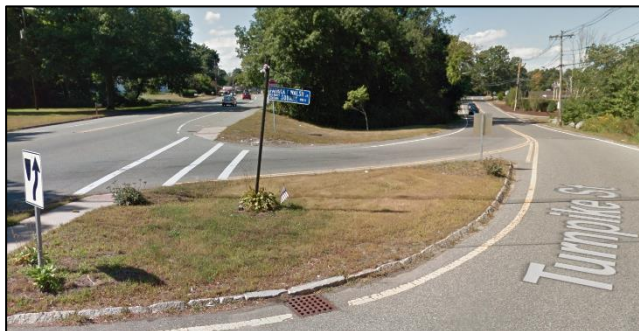
Sign on the traffic island dedicating Patrick Walsh Square has been hit by vehicles encroaching on the traffic island.
