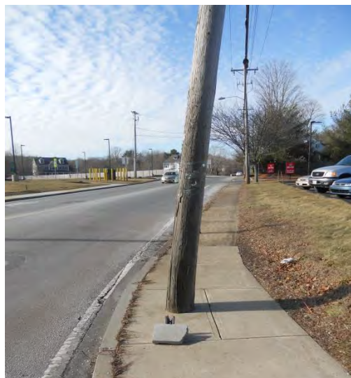
Missing Sign Post and Damaged Pole
