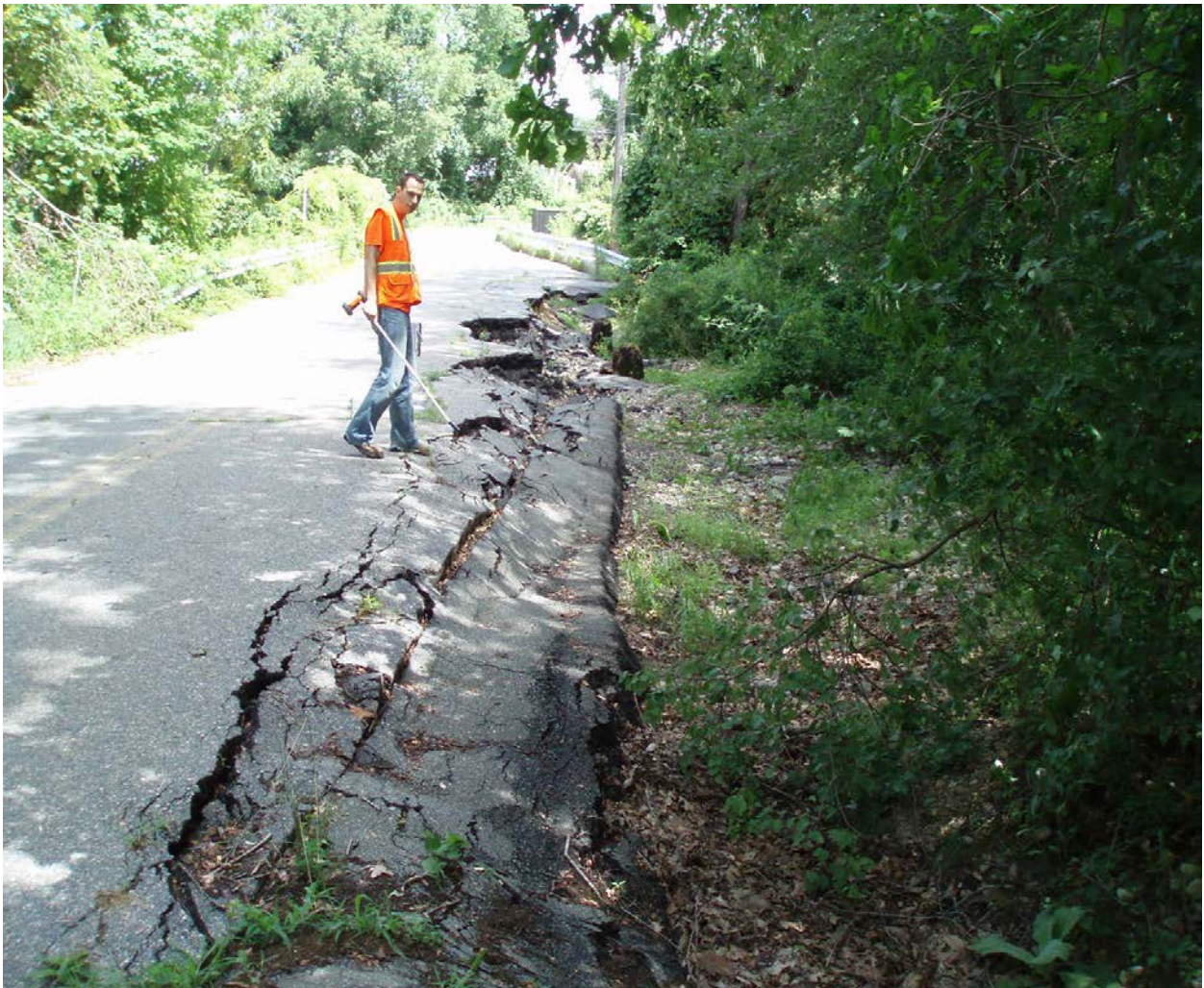
Figure 5: Bridge Street collapsed section
