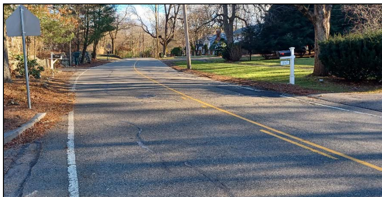
Photo above shows the Double Yellow Center Line (DYCL) faded and resembling a passing zone.
