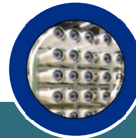
Reverse Osmosis Membranes
