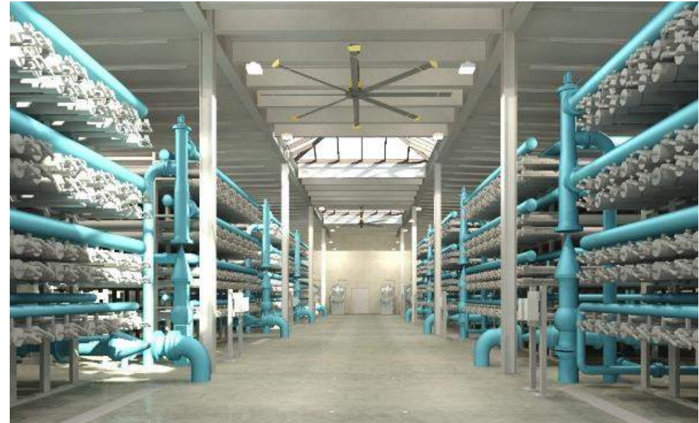
Brunswick County, NC Surface Water Treatment RO Facility (41-mgd capacity)
