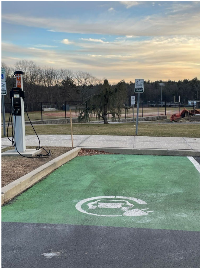
Figure 16: EV Charging Station
